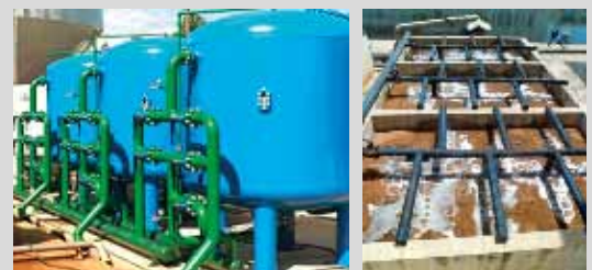
Sand filter system
